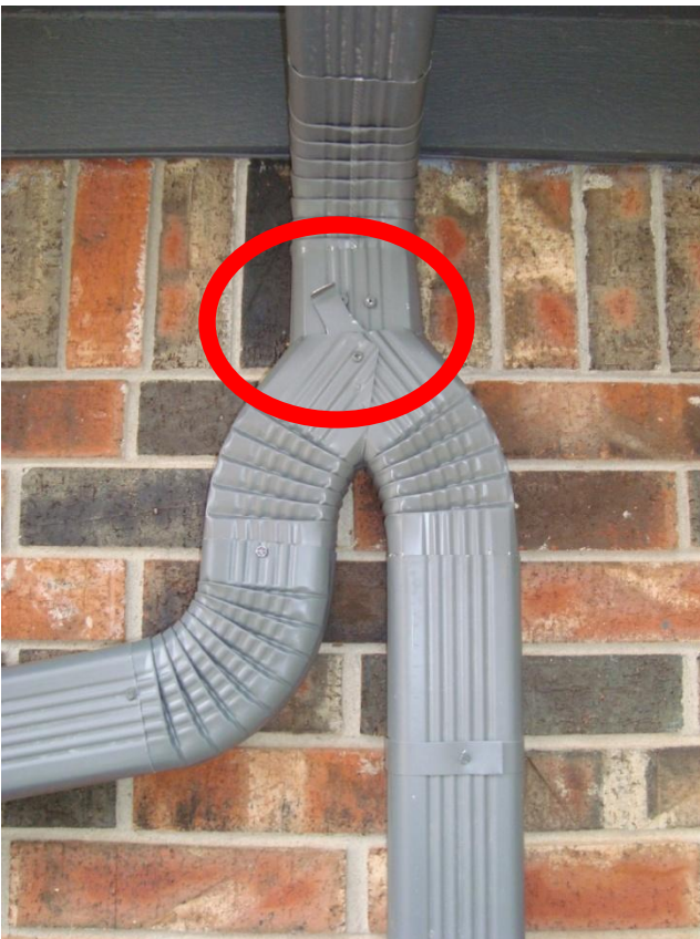
Y-shaped diverter section in 3" x 4" downspout. Lever diverts water either toward barrels or underground drain.
